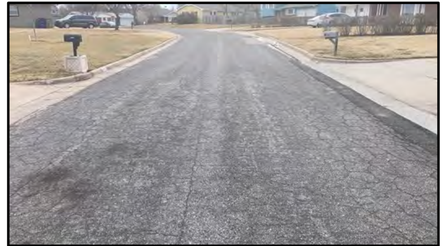
EXTENSIVE BLOCK CRACKING
